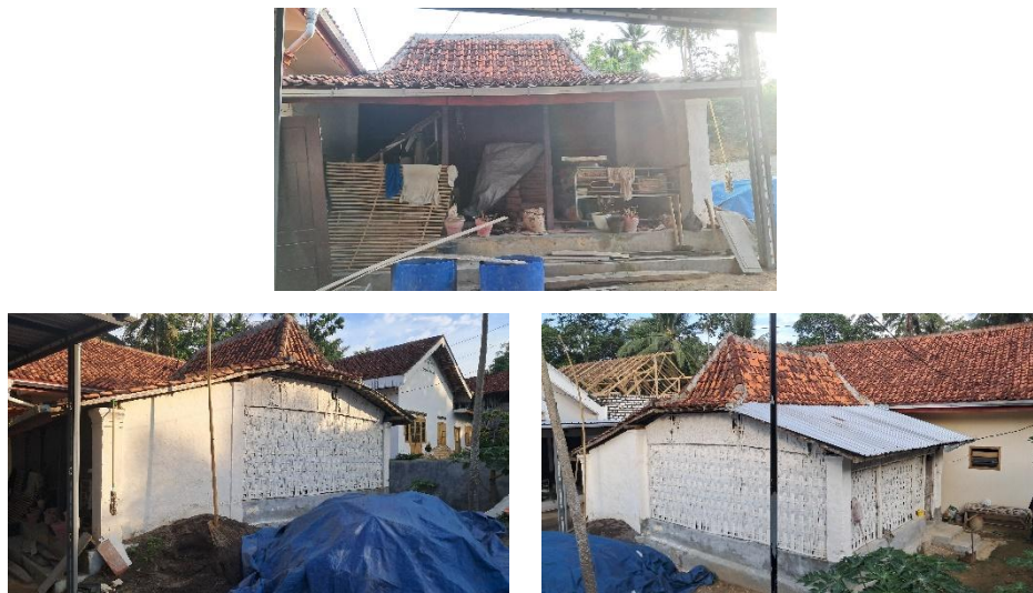
Figure 7. Front, side, and back views of Mr. Subahri's house (Source: Personal document)
