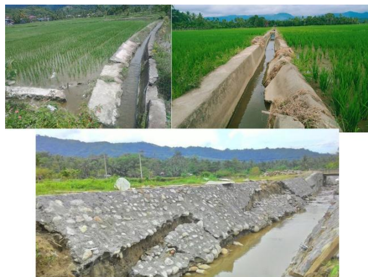
Fig. 1. Damaged Irrigations in Indonesia
