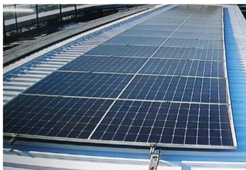
a) 18,36kWp PV rooftop
