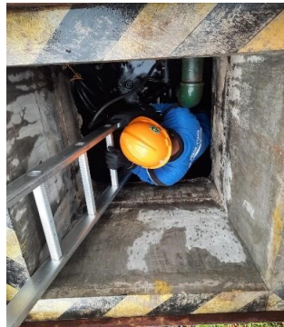
Gambar 1. Kondisi Pekerja Saat Memasuki Confined Space Groundtank Plant A1 PT.X
