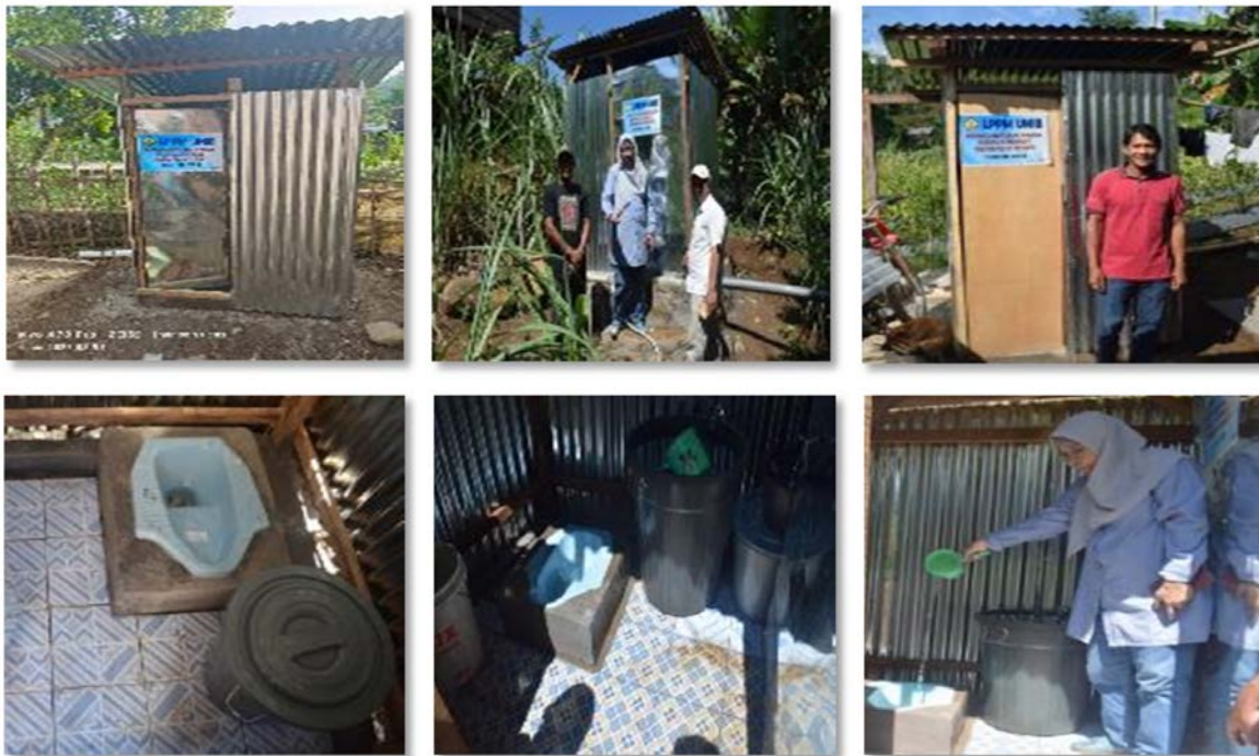
Figure 7. Construction/external and internal appearance of the toilets/WC (Results of LPPM UNIB Service)
