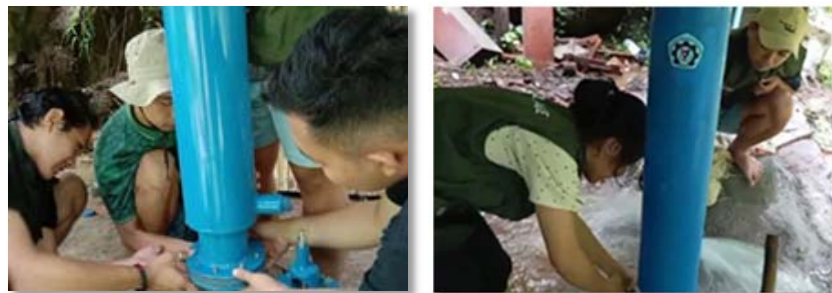
Figure 6. Testing and installation process of the hydram pump
