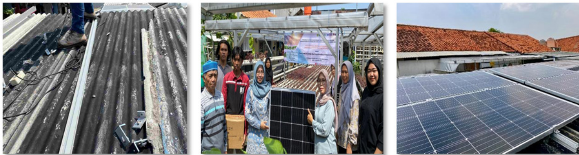
Figure 5. Solar panel installation program, existing condition of the roof of the partner warehouse (before), team and partner's, and 800wp solar panel installed on the roof (after)
