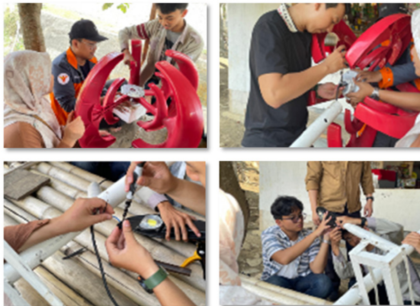
Figure 8. (a) Blade installation; (b) Blade assembly with rotor and generator; (c) Lamp cable assembly; (d) Lamp assembly with VAWT
