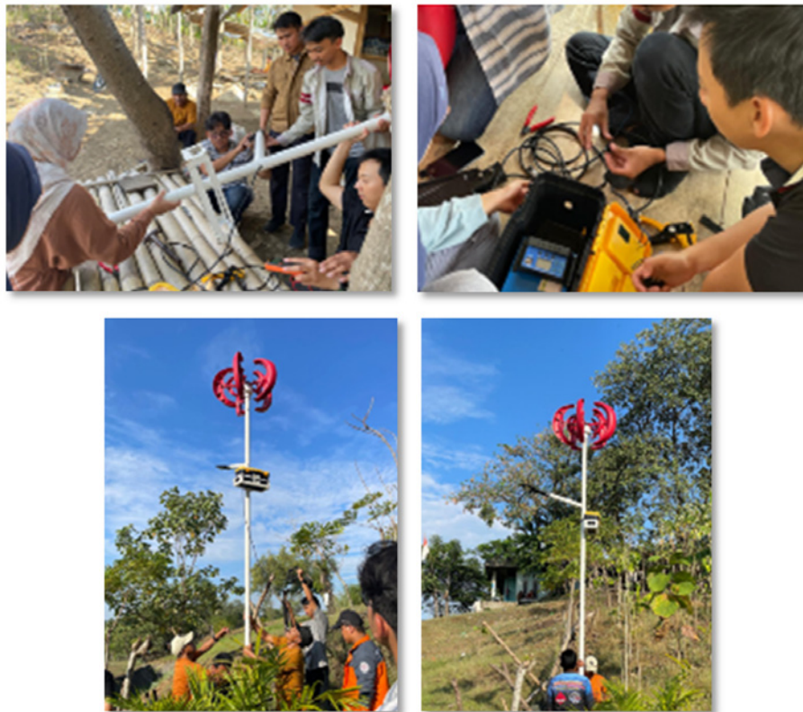
Figure 9. (a) Installation of PJU cables to poles; (b) Installation of power transmission systems; (c) Installation of VAWT and PJU; (d) Validation of system performance of installed PJU
