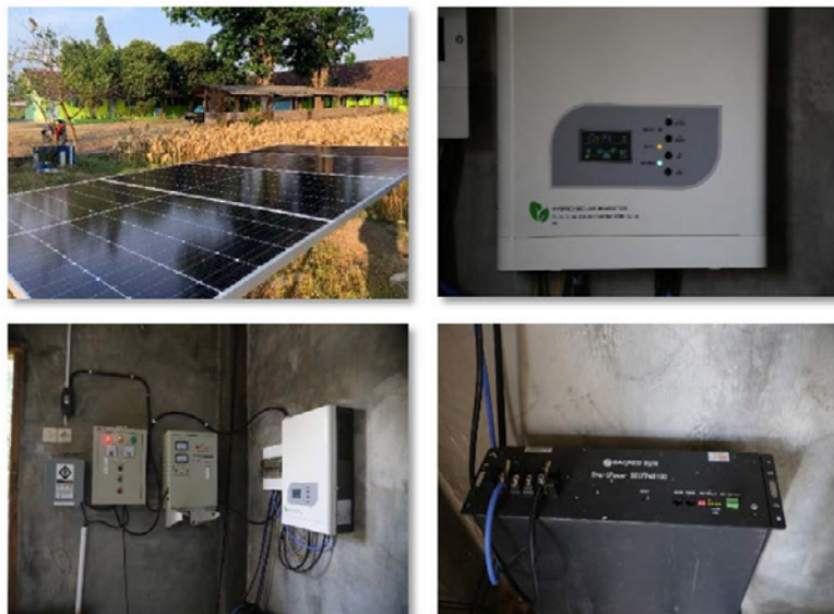
Figure 5. The components of the installed power generation system
