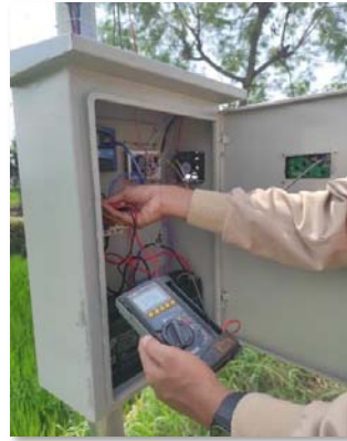
Figure 7. Checking the components and devices used in land monitoring equipment
