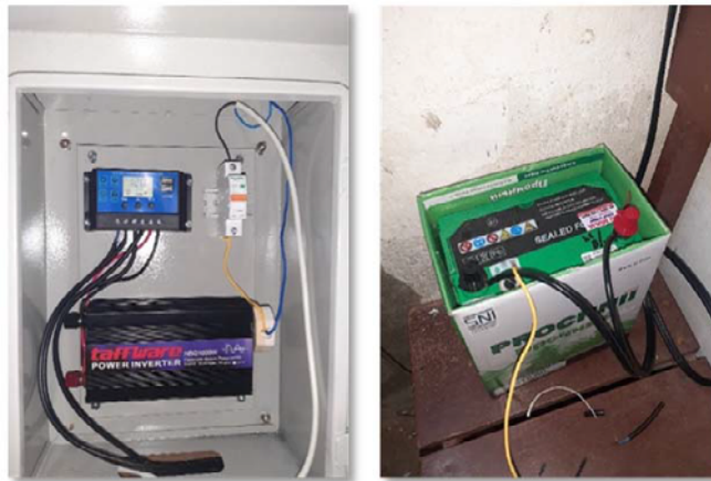
Figure 2. shows the testing of the inverter and system load simulation during the pre-installation phase Figure 3. captures the actual field test at the mushalla , including panel voltage measurement, SCC and battery setup, and the mushalla lighting powered by the system
