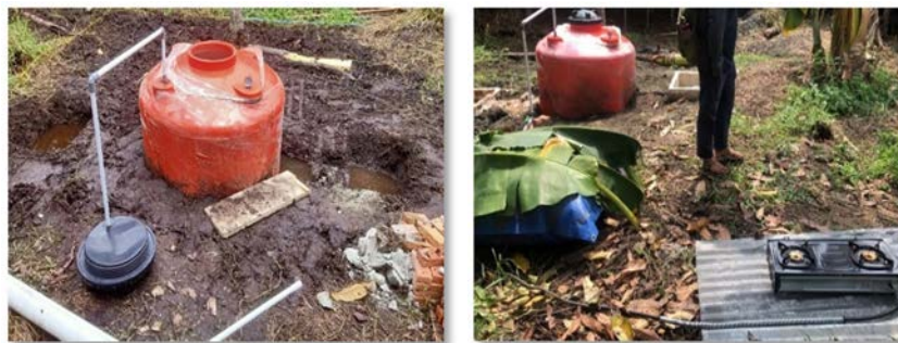
Figure 7. Illustrates the installation procedure for biogas processing using a biodigester installation Figure 8. Biogester installation complete installed and tested
