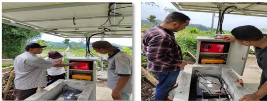
Figure 8. Inverter and SCC module test
