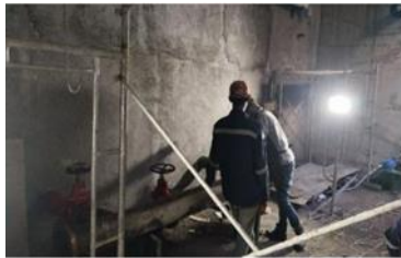
Figure 2.1 Ground Water Tank(GWT)
