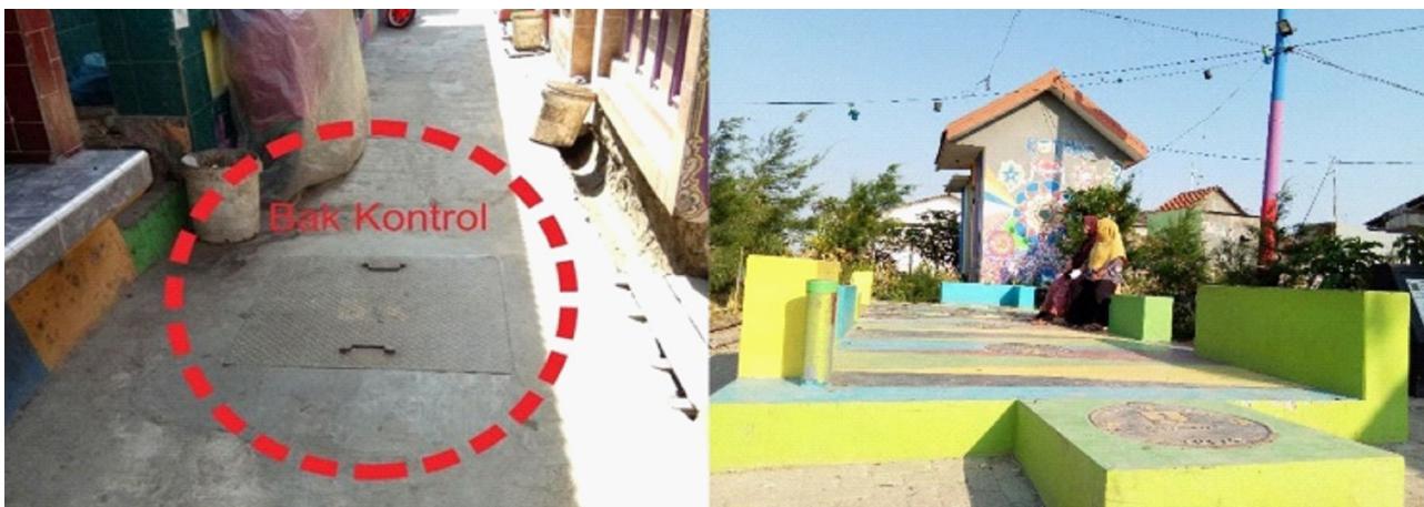
Figure 13. Drainage Control Tubes and WWTPs
