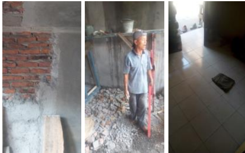
Figure 5. Different materials used for raising and waterproofing on the floor and the walls. (Source: taken from the site 22 Oct 2019)
